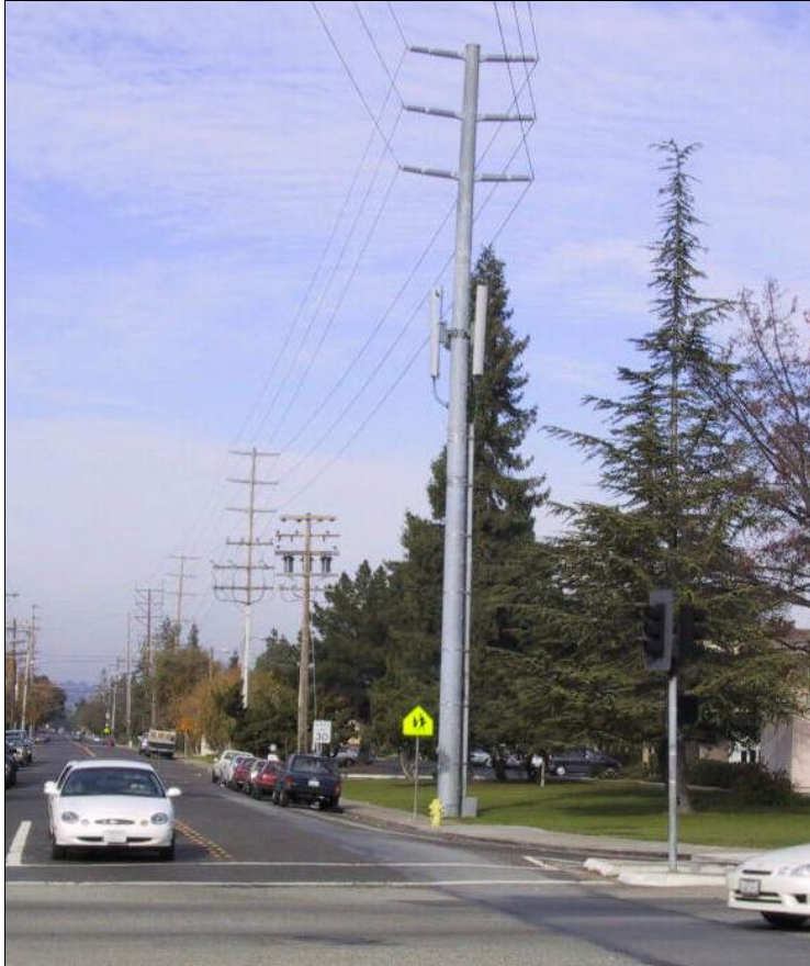
Figure 40 - Directional Antenna Site on Power Pole
