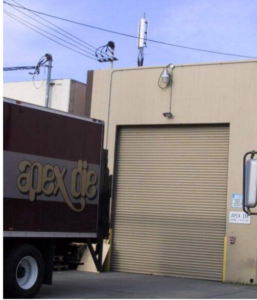
Figure 38 -Directional Antennas On One Story Building
